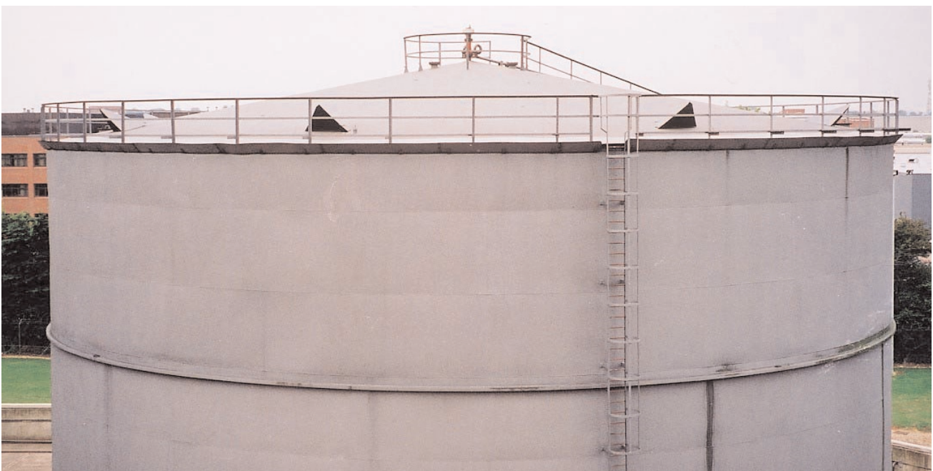
Figure 3 Tank top details before the incident
