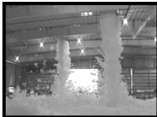
CEILING MOUNTED HIGH EXPANSION FOAM GENERATORS, SHOWING TOTAL FLOODING
