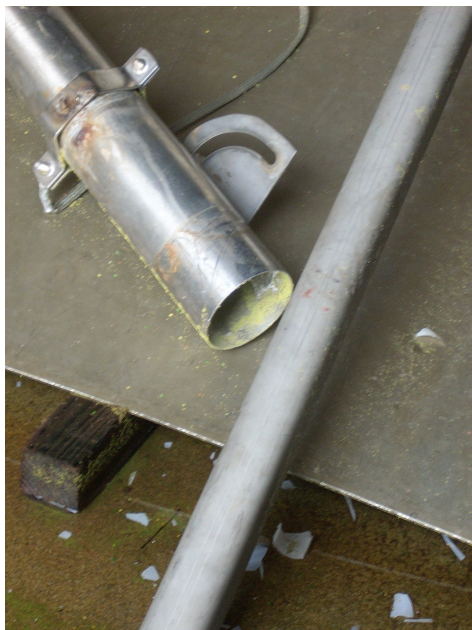
Metal debris, from the pipe blasted by the explosion, found on the floor. The picture on the left shows residue from pyrotechnic dust (yellowish) covering the inner pipe wall.
