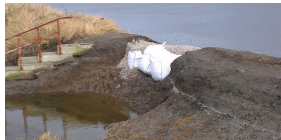
Figure 3 : Breach in flood defence with temporary staunching, source Inter Terminals
