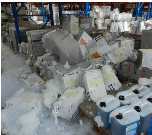
Figure 3 : Cell 1 after activating the foam extinction (Source Operator - ARR)
