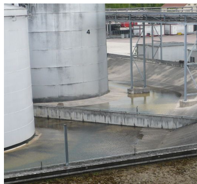
Retention basin for an unsealed tank (Source: DREAL Champagne-Ardenne)
