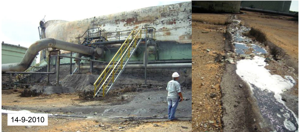
Figure 6 The situation near the burnt naphtha tank after the fire. Debris, probably of oil, water and foams, have leaked from the tank to the premises. Photos taken in the week of September 14, 2010.
