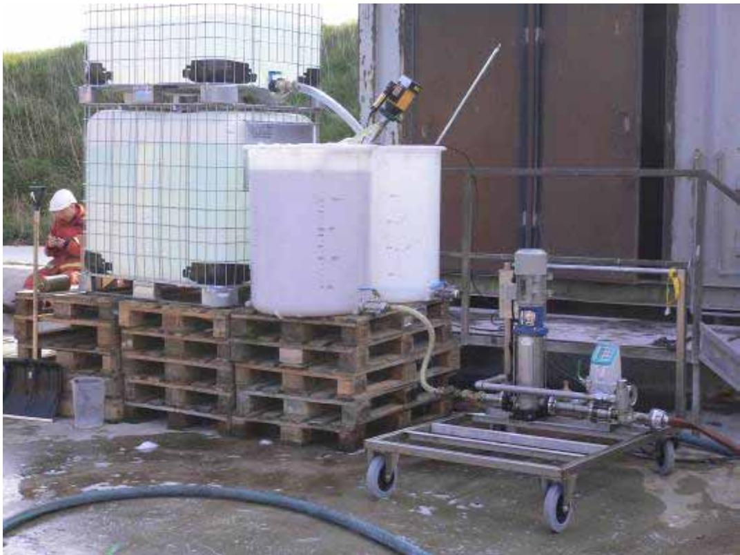
Photograph 4: Pre-Mix Vessels and Pump Skid
