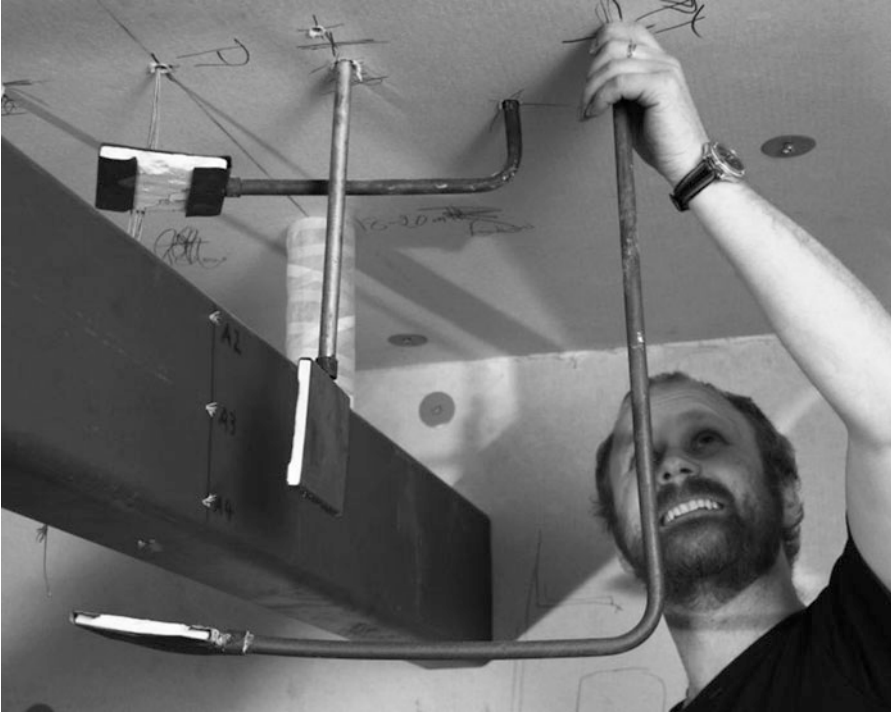
Fig. 34.4 Plate thermometers being mounted around a steel girder for measuring local thermal exposures. Note that the plate thermometers are mounted so that the front
