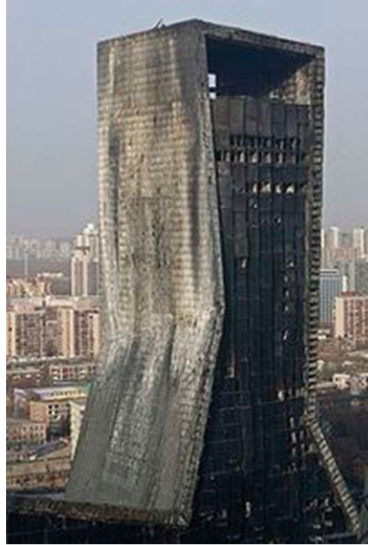
Fig. 86.26 Exterior condition of building after fire (By BeiBar (panoramio) [CC-BY-SA-3.0 ( http://creativecommons.org/licenses/by-sa/3.0/ )], via Wikimedia Commons)
