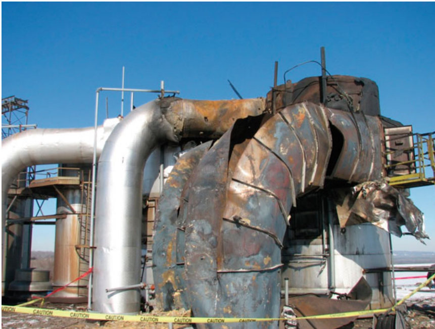
Fig. 70.10 Evidence of dust explosion and fire in cyclone collector and ducting
