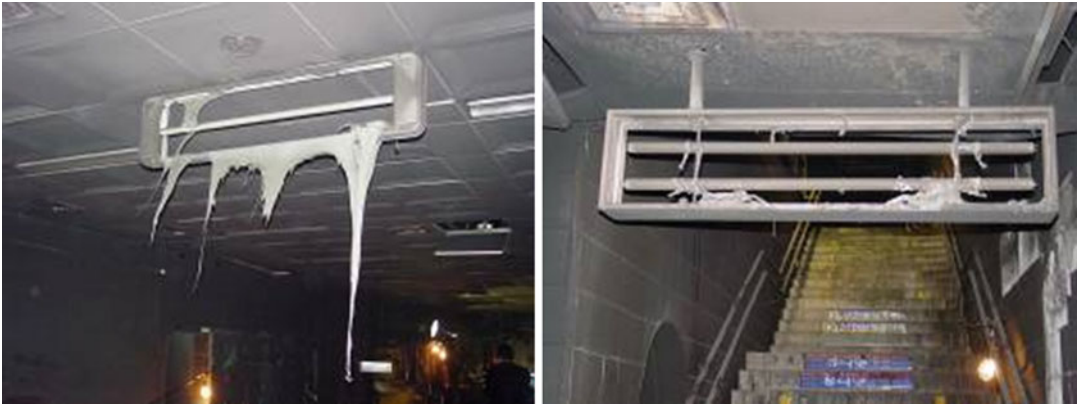
Fig. 61.14 Damaged emergency light in Daegu subway fire
