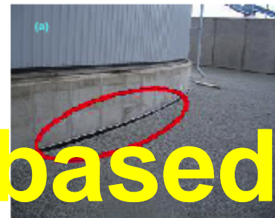
Right - Fig 2.3.2.1(d). Bund drain valves apart from those to remote containment basin should be normally kept closed
